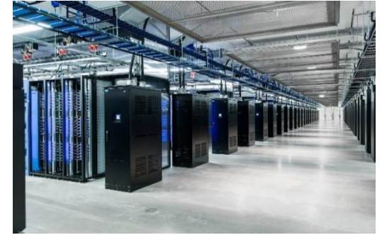
Data center campus projects, USA
